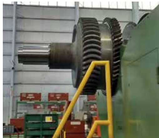
Mustang Station's combined-cycle unit experienced an unplanned steam turbine outage early in 2015. These photos show the submerged arc welding in progress and the steam turbine rotor after repair.
