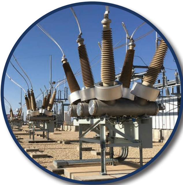
Top photo, construction of Elk Station Units 2 and 3 benefited from the experience gained when the team built Unit 1, with the result of a project completed ahead of schedule and under budget. Bottom photo, high voltage circuit breakers in the Antelope Station switchyard provide a critical element of protection and reliability.
